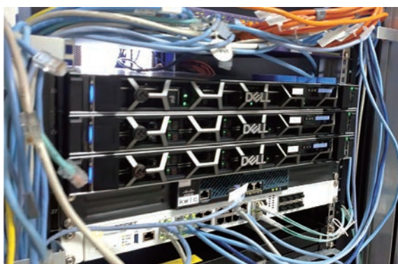
演習室用サーバ Servers for Practice Rooms
