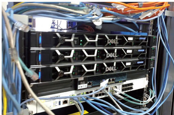
演習室用サーバ Servers for Practice Rooms
