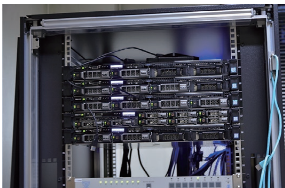
演習室用サーバ Servers for Seminar Rooms
